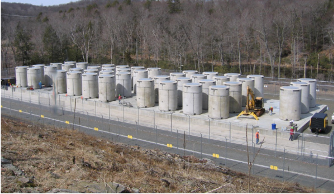
Figure 2.2: Connecticut Yankee Dry Cask Storage Facility. If CT Yankee had been a coal plant and we tried to store the coal waste on the same pad, it would be a column 7000 feet high.
